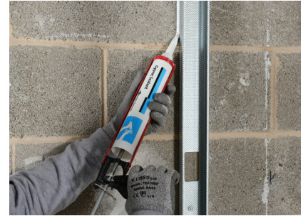
The perimeter of the partition is then sealed on both sides with Gyproc Sealant.
