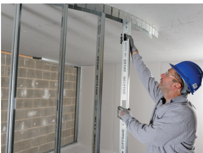
Gypframe studs are fitted and fixed into the Gypframe 72 EDCL 80 Curvellyner Channels at the required centres.
