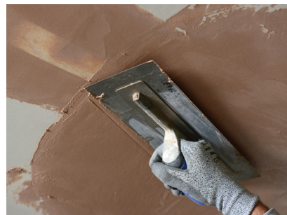
For best results Gyproc plaster is applied with firm pressure, built out to the required thickness in two applications and trowelled to a smooth matt finish. Good site practice should be followed, as outlined in BS EN 13914 - 2: Design Considerations and Essential Principles for Internal Plastering .
