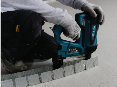
Gypframe 72 EDCL 80 Curvellyner Channels are suitably fixed to the floor and soffit, bent by hand to suit the required radius.
