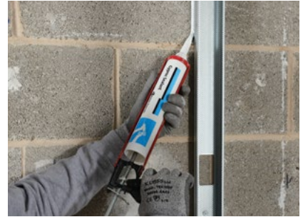
The perimeter of the partition is then sealed on both sides with Cyproc Sealant.
