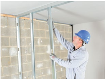
Gypframe studs are then friction fitted into the Gypframe Deep Flange Floor & Ceiling Channels at required centres.
