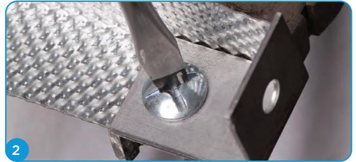
2 Form hangers by securing Gyframe MF8 Strap Hanger to Gyframe MF12 Soffit Cleats with Gyframe MF11 Nuts and Bolts.
