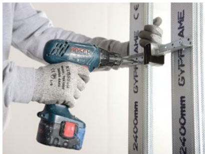
The Gypframe 92 S 10 'C' Studs are then braced together in pairs with either staggered Gypframe GAB3 Acoustic Braces,
