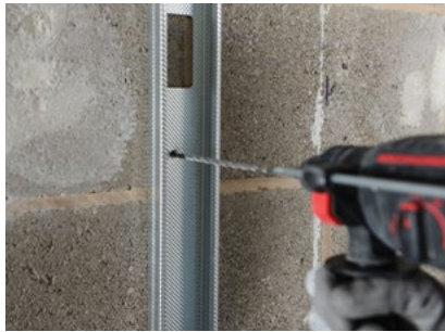
Gypframe 92 S 10 'C' Studs are fixed at abutments and door openings in two rows.
