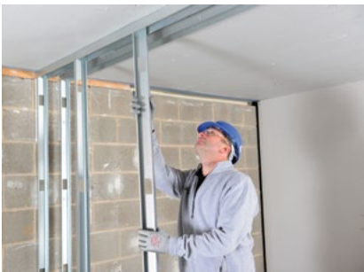
Gypframe 92 S 10 'C' Studs are then friction fitted into the Gypframe Channels at the required centres, and door openings are constructed to the Heavy and Severe Duty Rating door detail.
