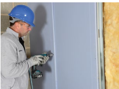
When applying multiple layers of board, ensure that all board joints are staggered on both sides of the partition.
