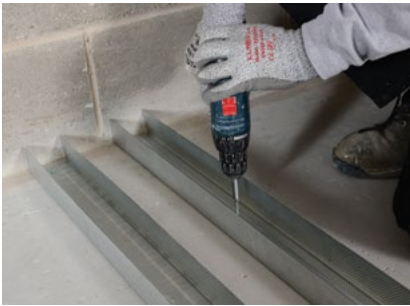
Gypframe Floor & Ceiling Channels are suitably fixed to the floor and soffit in two rows.
